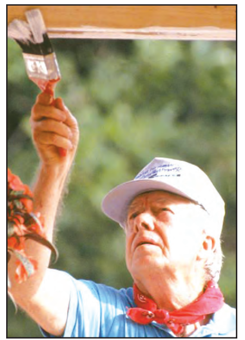
President Jimmy Carter paints one of the many Habitat for Humanity houses he helped to build.
