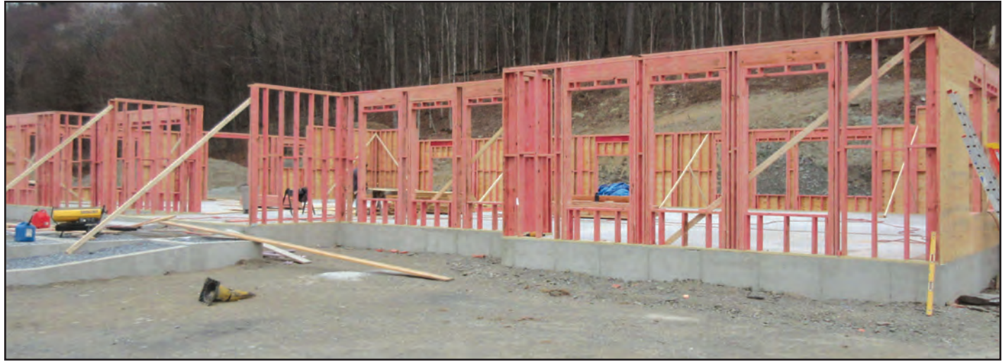
The first floor framing is in place at the new school building at Upton Lake Christian School in Clinton Corners.
