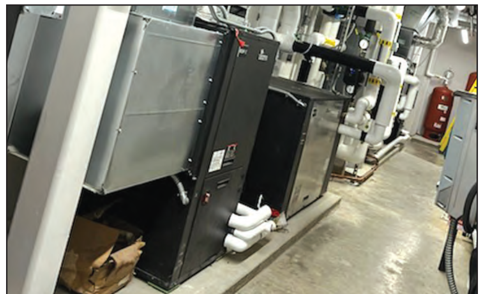
The renovated firehouse in the City of Beacon, on Wolcott Ave., has energy-efficient systems and green building materials.
