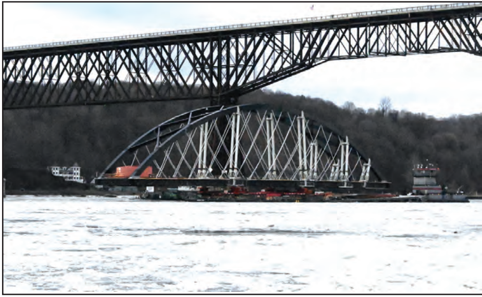
A new railway bridge section for the Portal North Bridge across the Hackensack River in New Jersey passes under Poughkeepsie's Walkway Over the Hudson Bridge on Jan. 15 en route to its new home. Photo by Jim Donick
