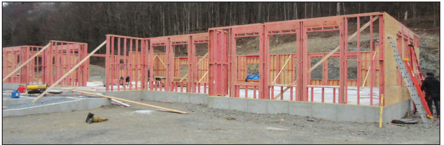
The first floor framing is in place at the new school building at Upton Lake Christian School in Clinton Corners. Courtesy photo
