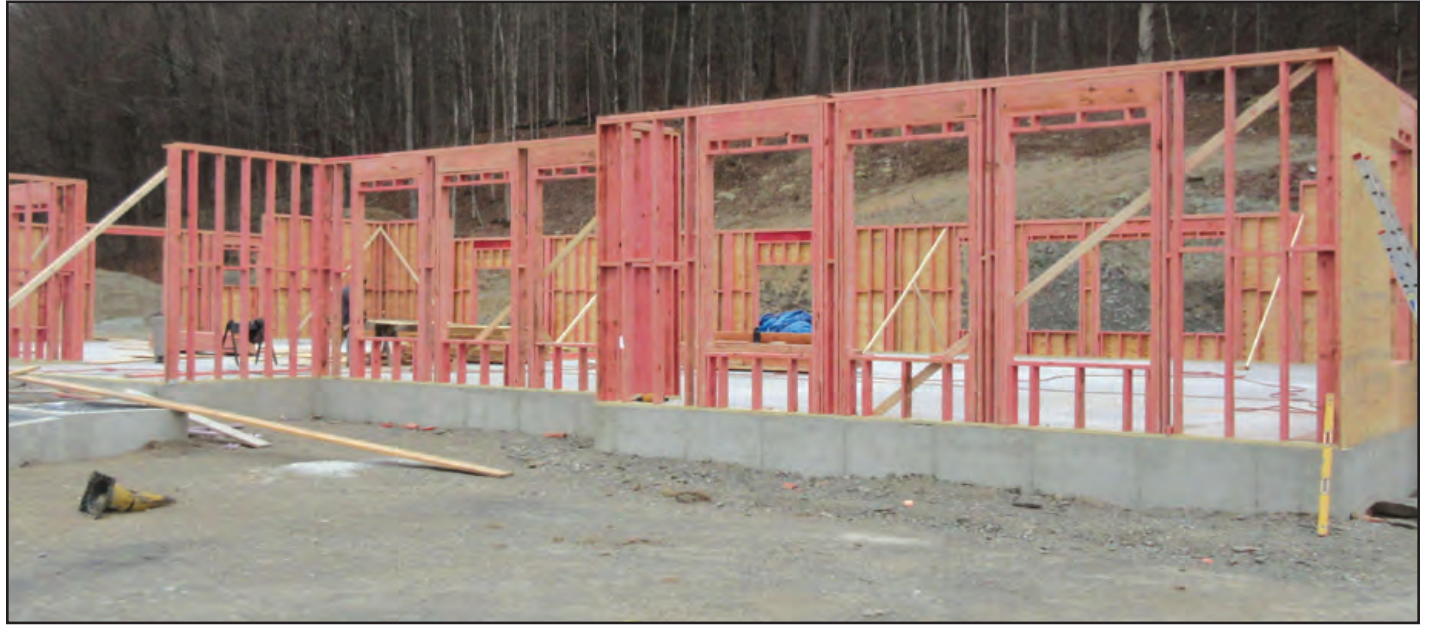
The first floor framing is in place at the new school building at Upton Lake Christian School in Clinton Corners.
